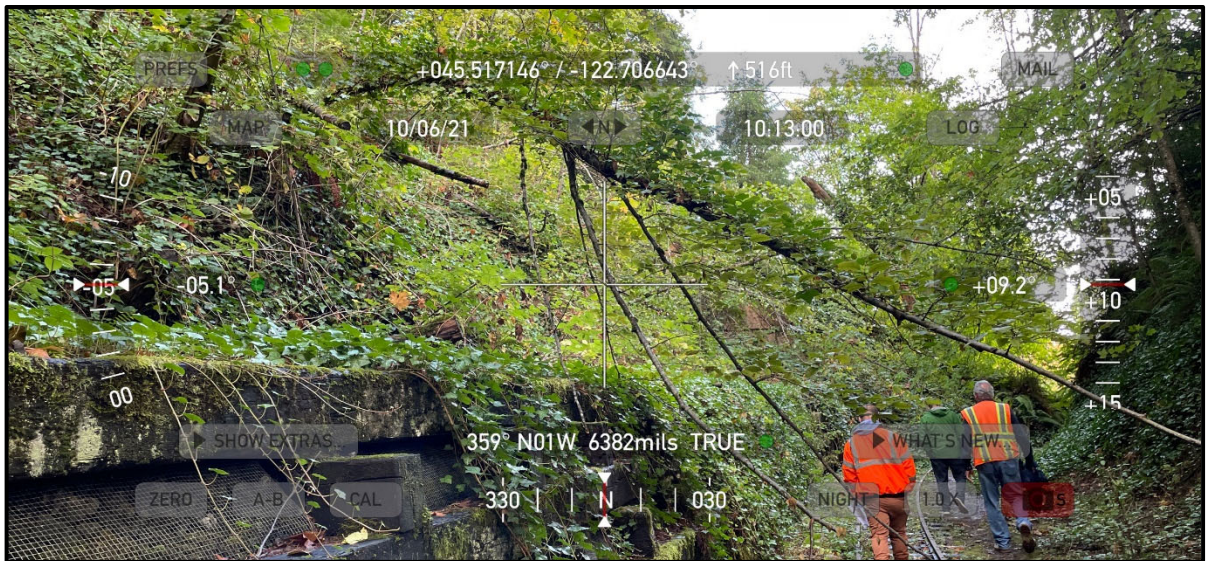
Photo TH000026: Area near 1997 landslide looking north (appr. STA 56+00 to 57+00)
