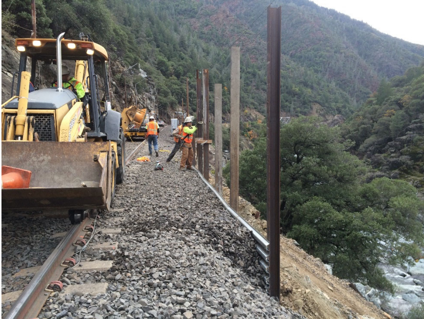
Exhibit 6-1: Installation of a soldier pile wall used for railroad embankment support on steep slope on a rail alignment in California
